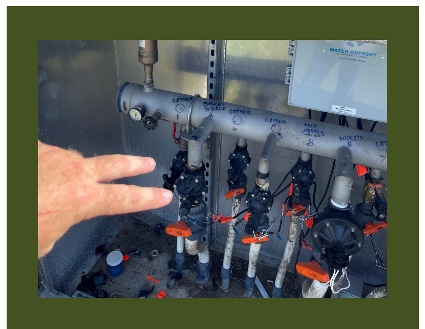
HICKORY RIDGE COMPUTER CONTROLLER INSTALLATION
